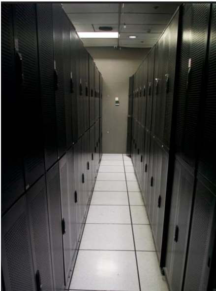
Fasilitas Data center TIFA 1
