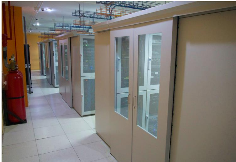
Fasilitas Data center
