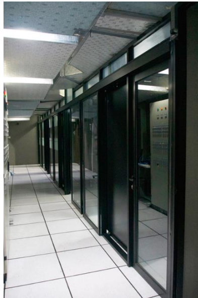
Fasilitas Data center TIFA 2
