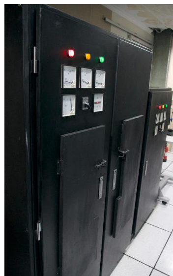
UPS (Uninterruptible Power Supply)
