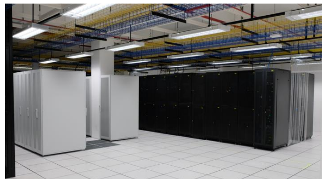
Fasilitas Data Center
