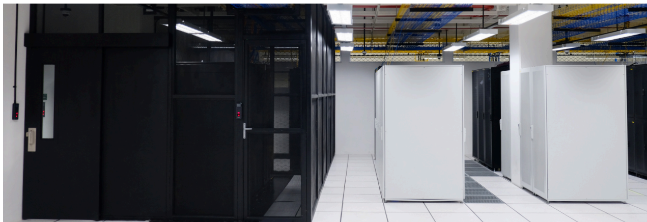
Data Hall 1 AREA31
