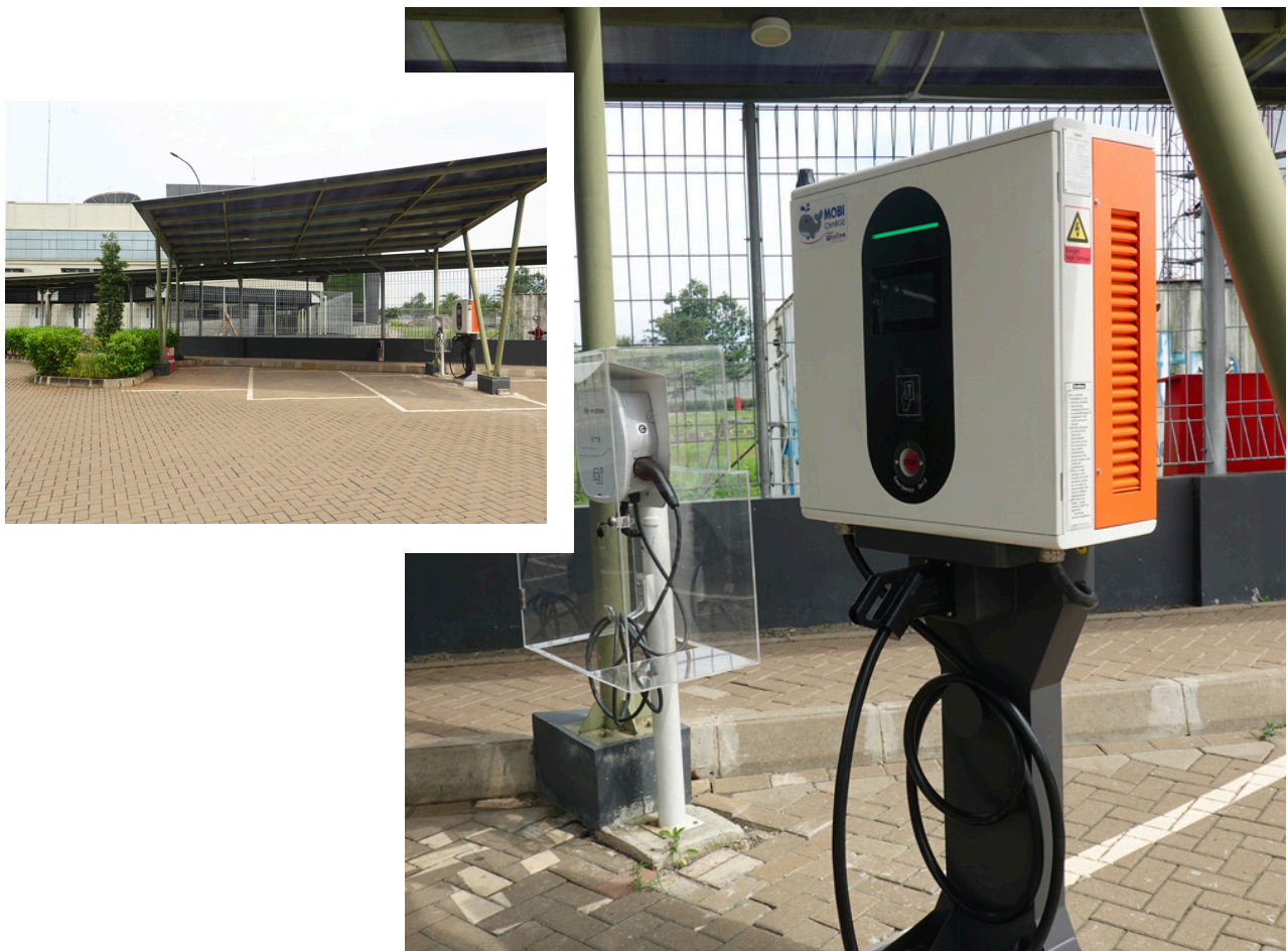
EV Charging pada lahan parkir AREA31 EV Charging at AREA31 parking lot
