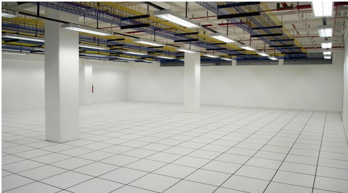
Data Hall AREA31
