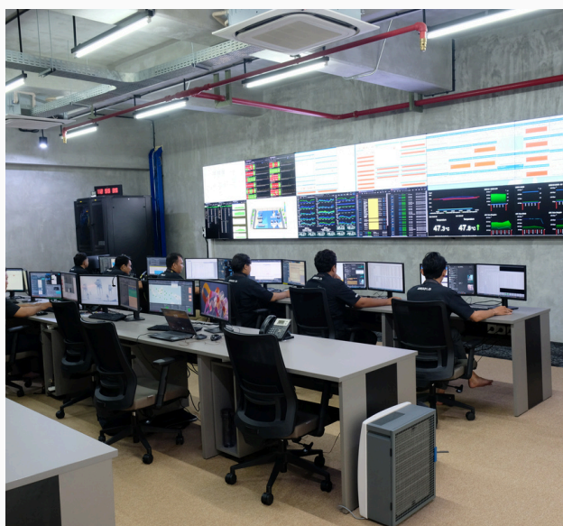
Air Purifier pada ruangan Command Center AREA31 Air Purifier in the AREA31 Command Center room
