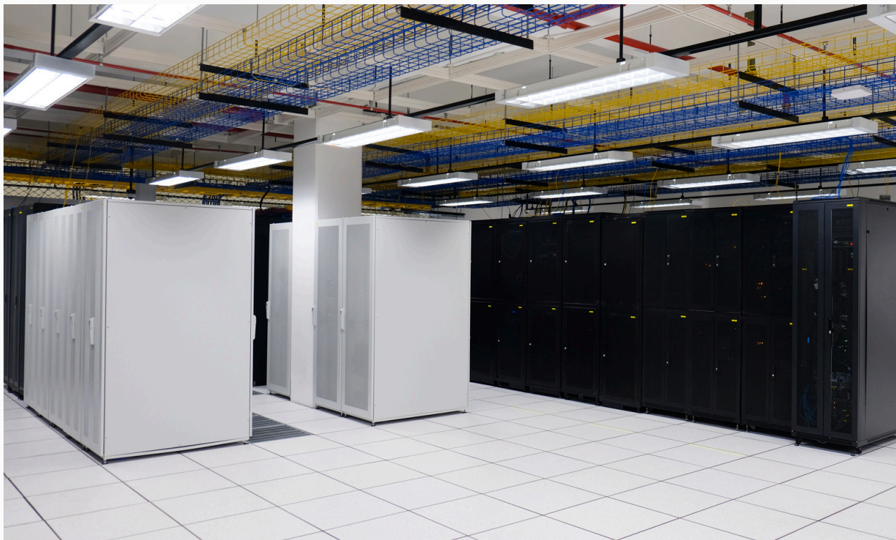
Data Center AREA31 Cyber
